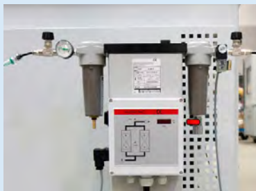
Additional Drying Capacity
